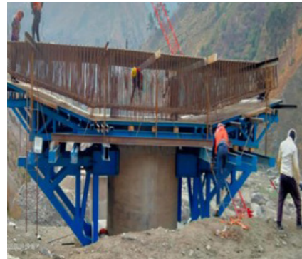
Construction of Four Laning of part of Ramban to Banihal Section of NH-1A (Now NH-44)
